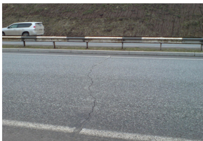
Fig. 5. A transverse frost crack in the middle of excavation
