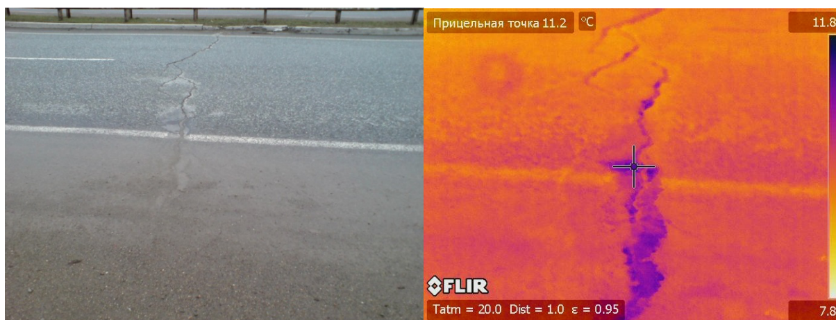
Fig. 4. View and the programme cracks in the plot mound – excavation
