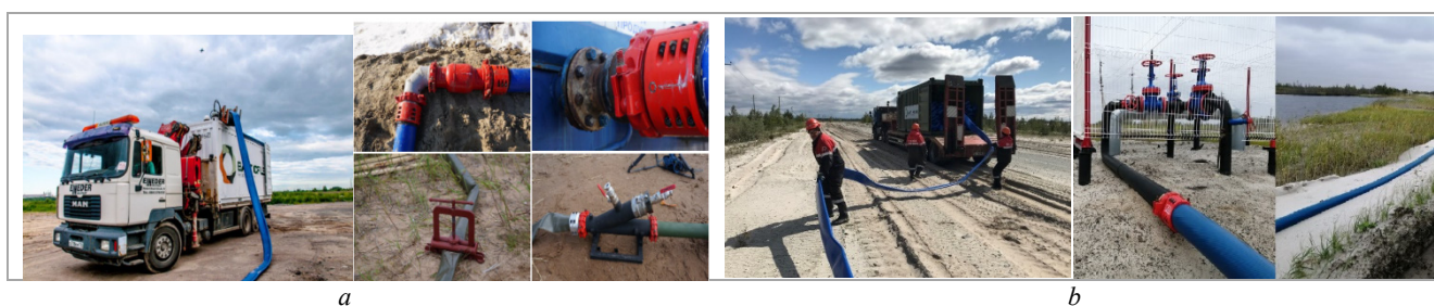
Fig. 6. Mobile technical stations : a – external view of mobile technical station and connections in portable pipeline; b – station assembling with the connection with existing infrastructure
