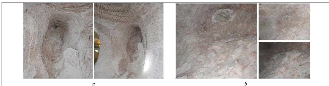
Fig. 3. Cavity form appeared after the sudden destructing the marginal massif: a – in the wall of the exploratory drift No. 2; b – in the face of the transport drift No. 1
